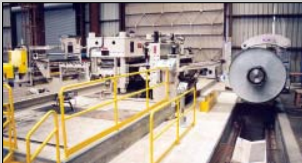
60,000# x 72" Multi-Blanking Line Entry Section
